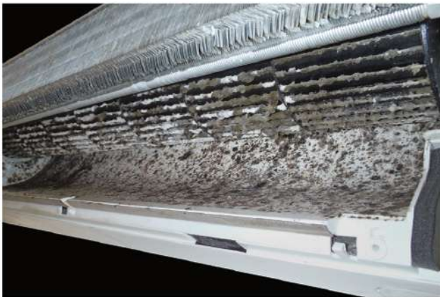
Mini-Split blower with MOLD
